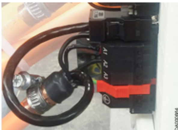
Fig. 95: Encoder cable forming a loop to be led to connection point XG20
